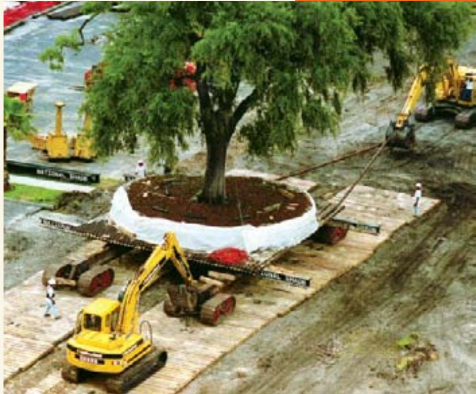
Two large tractors were needed to carefully tow the trees about 75 yards to new homes.
